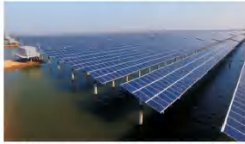
Photovoltaic Power Project
